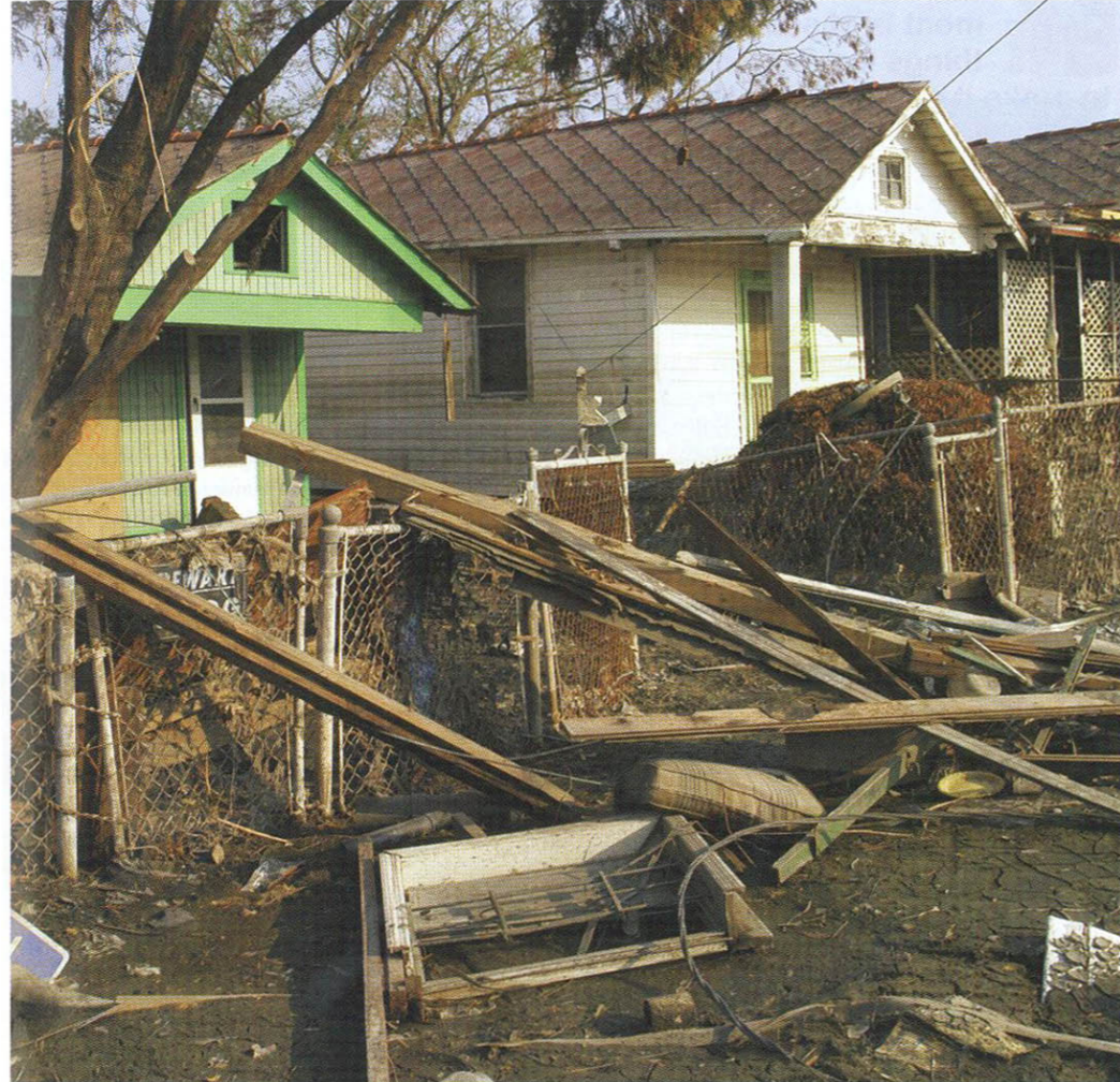
HARD HIT: Hurricane Katrina's devastation shows the need for tougher building standards.
